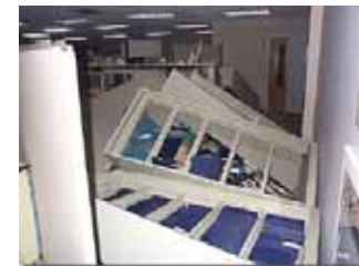
This example of non-structural damage is common after earthquakes of even moderate size - © FEMA File Photo
